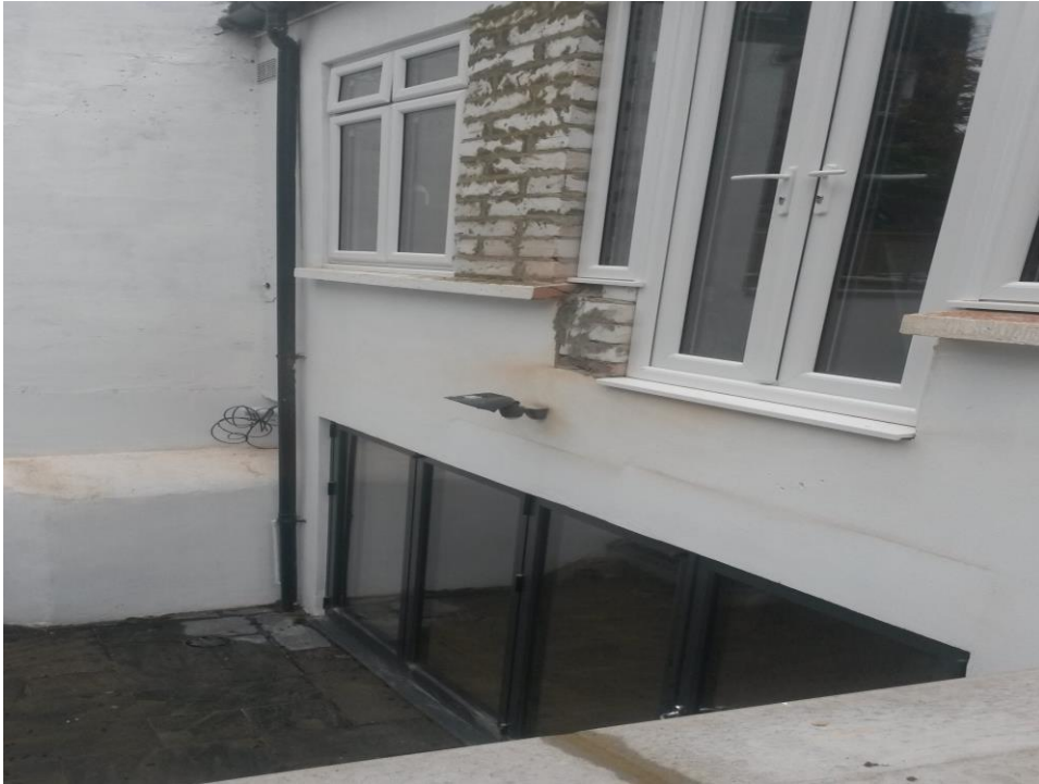
Photo 5: View of the existing full width 2 storey rear extension at ground and basement level to adjoining neighbour No.354 Caledonian Road.
